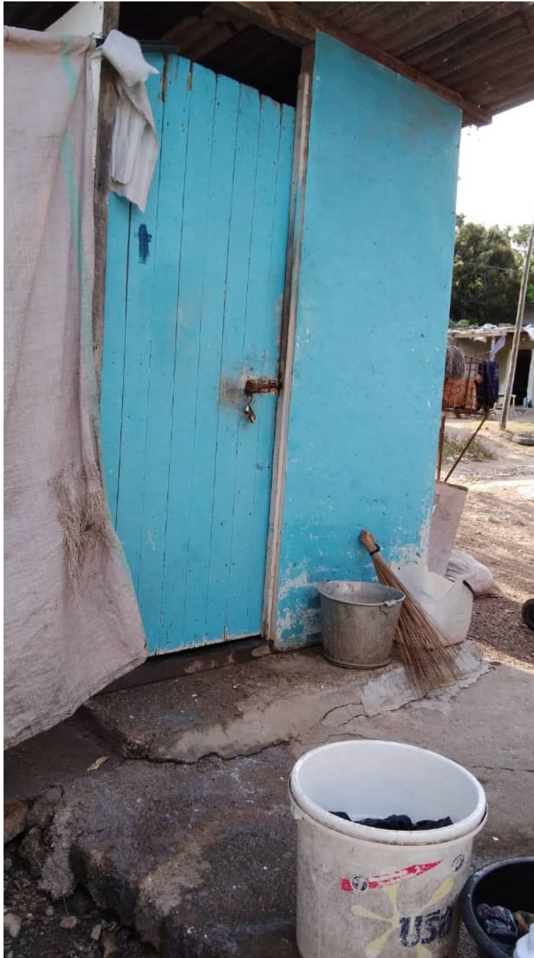
This is the first septic tank toilet built in Pari village. It was built 40 years ago and is still functioning.
