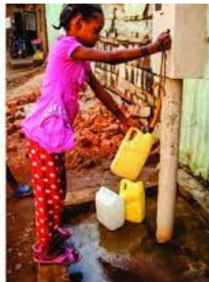
Prepaid tap stands are easy for children to use. Recent models include solar panels.
