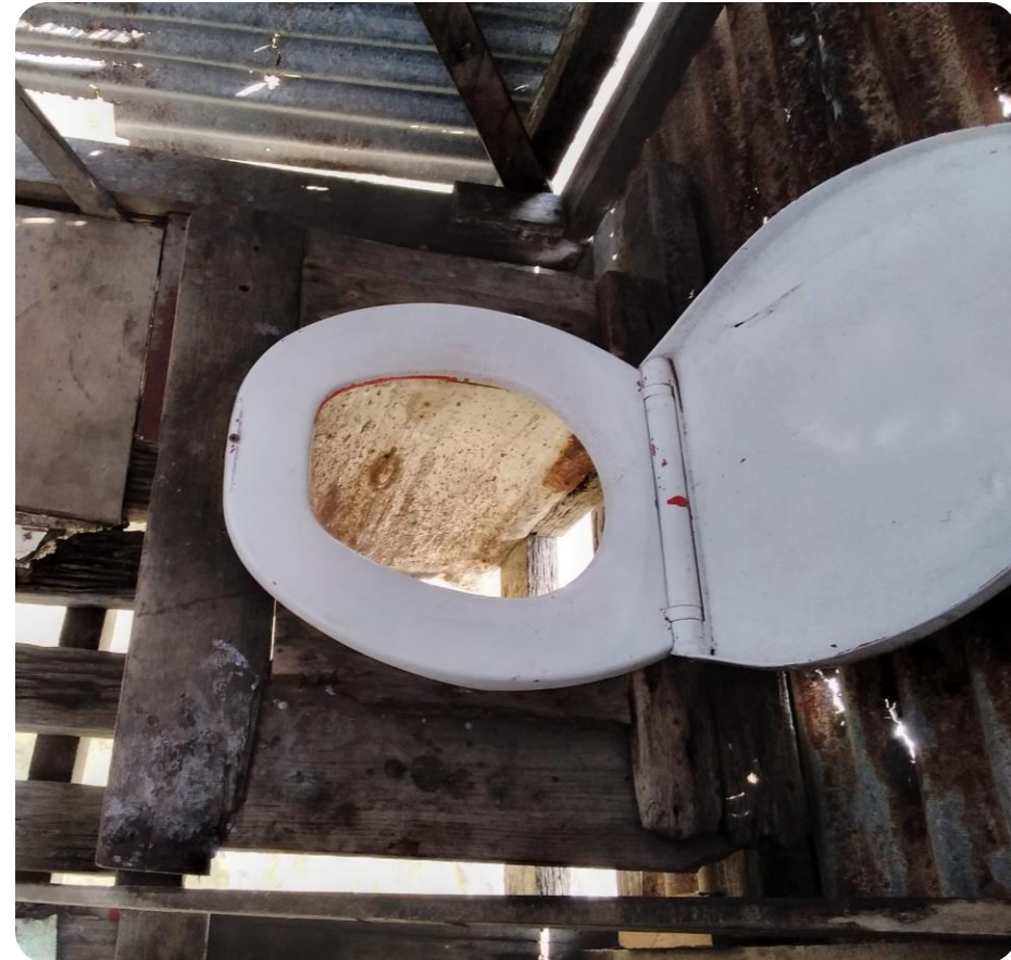
Inside Hanging toilet, Pari Village NCD
